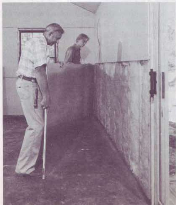
Gypsum board having one face covered with aluminum foil, shown here being installed horizontally, provides an interior wall with a vapor barrier.
